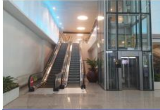
Escalator and Elevator
